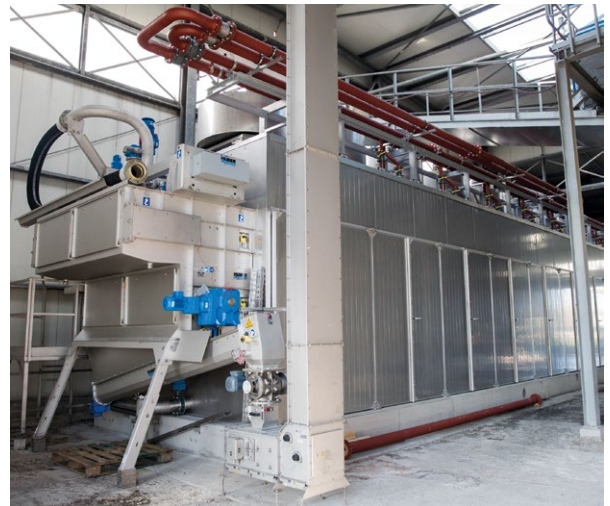
Belt dryer in the converted sludge drying plant
