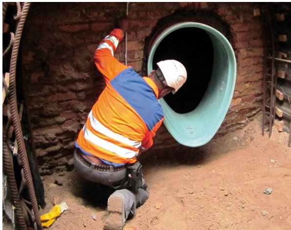
Introducing a plastic pipe into the main sewer using the lining/reinforcement method
