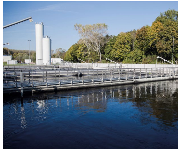
Powdered activated carbon system with two activated charcoal silos
