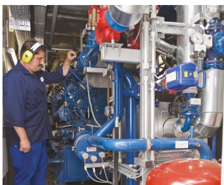
Gas motor in a container-housed CHP system
