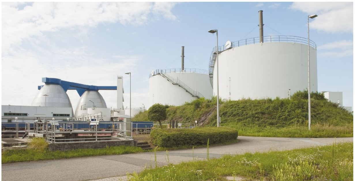
Generation and storage of biogas in digesters and gas holders
